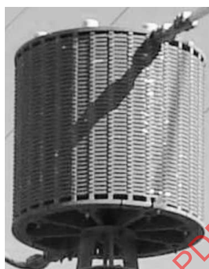
Figure 23 – HV line trap
