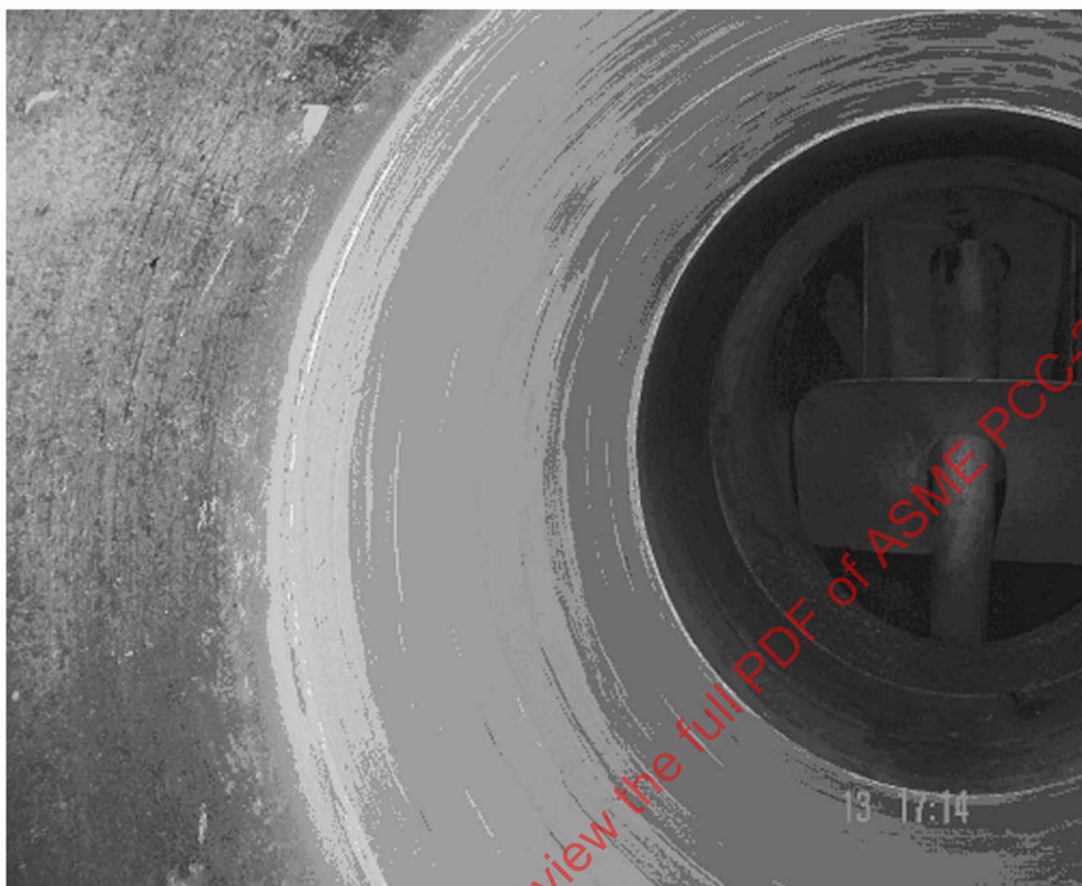
Figure 403-1.1-1 Structural Liner in Raw Water System
